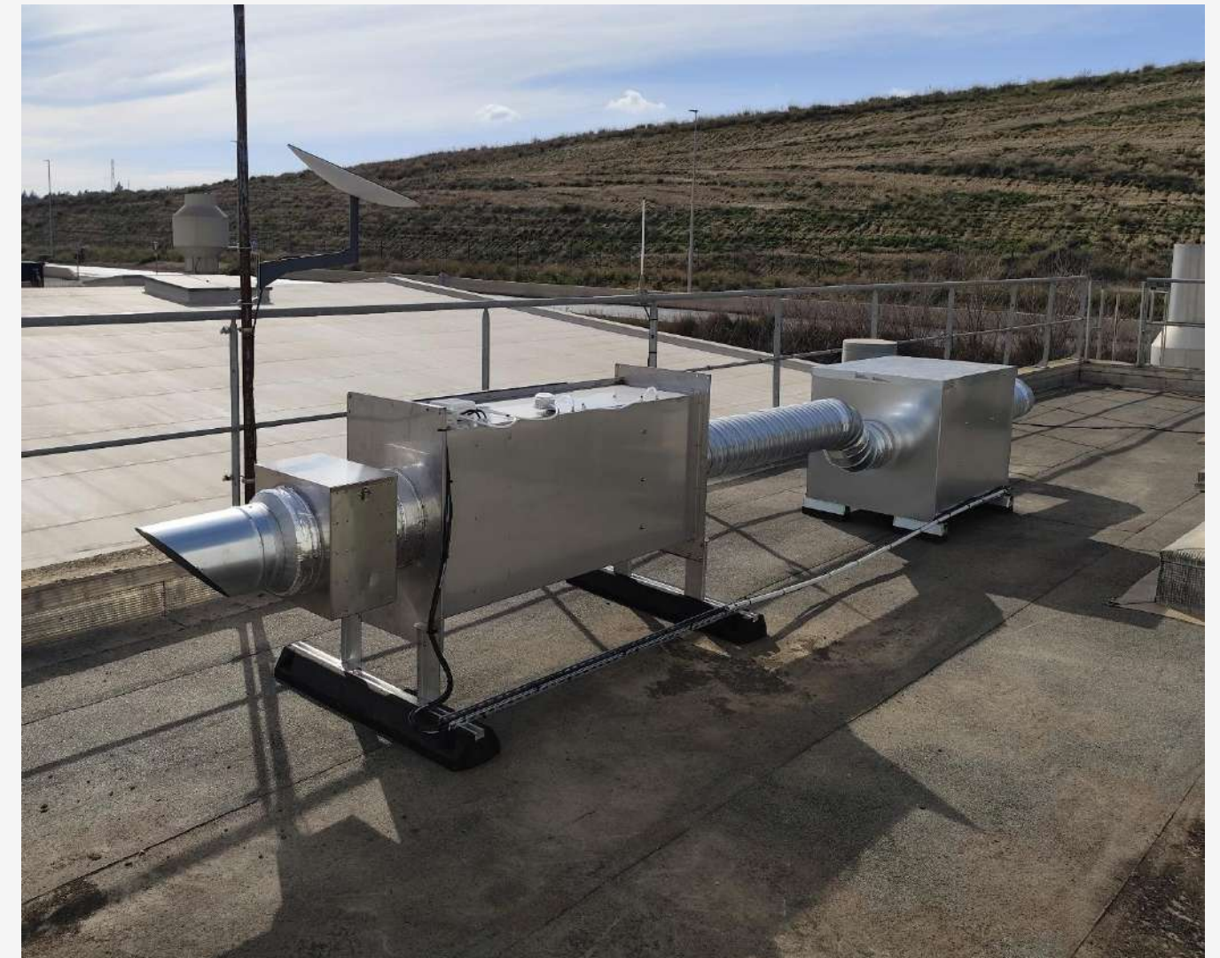
Example of a pilot installation
