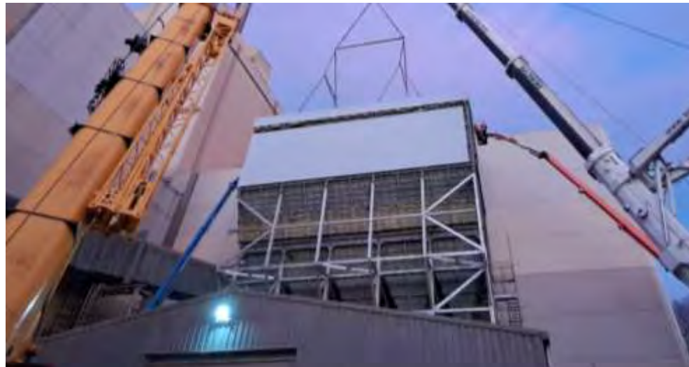
Figure 3 top view of Fabric Filter in Cauldon Lafarge plant, UK
