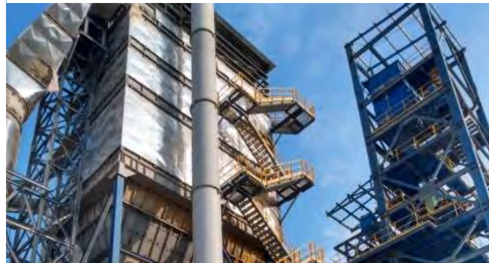
Figure 2 – Process Fabric Filter in the Yumbo cement plant, Colombia
