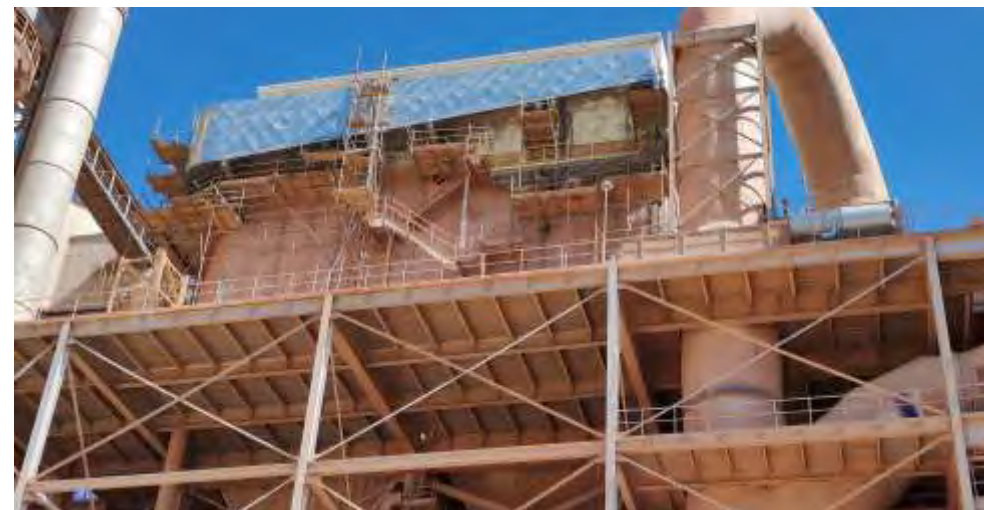
Figure 4 top view of Fabric Filter coal mill in Medcem plant, Turkey
