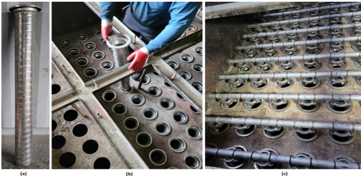
Fig.5. Industrial installation of the pleated SCR pellet catalyst filter bag system: (a) SCR pellet catalyst-filled cartridge, (b) bag filter chamber equipped with pleated SCR catalyst filter bags, and (c) low-pressure high-volume pulse injection valve bundles for off-line bag cleaning.
